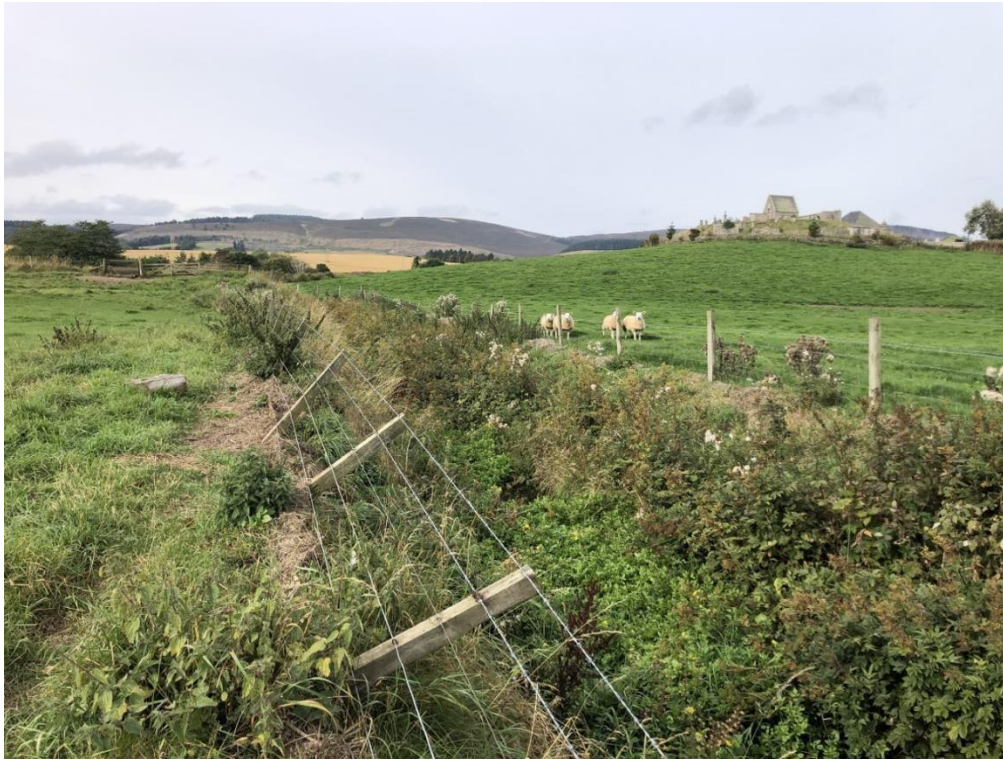
Figure 4.20 Fence line undermined by bank erosion on the river right bank of the Auld Water. This section of erosion is noted within the same field as the embankment breach.
