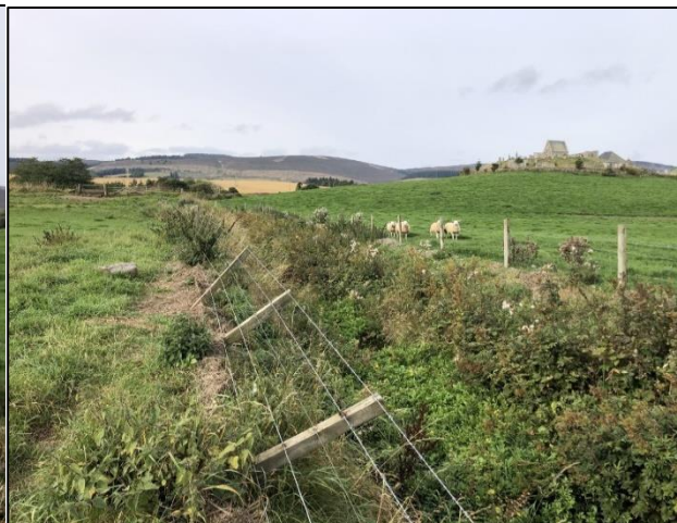
Figure 3.23 Collapsing fence line on the river right bank, indicating bank instability. It is recommended that this fence line is set back, the bank reprofiled and riparian zone planted.
