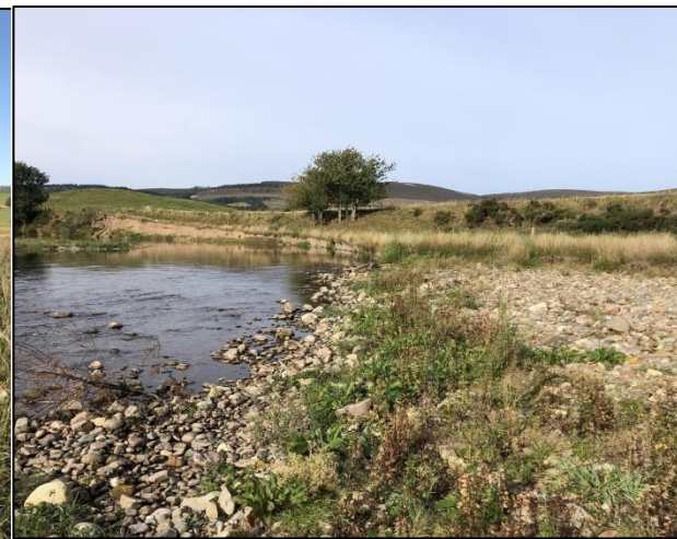
Figure 3.9. Looking upstream at the bank erosion, showing the low section of channel bank (~1 m high) at the embankment breach area.
