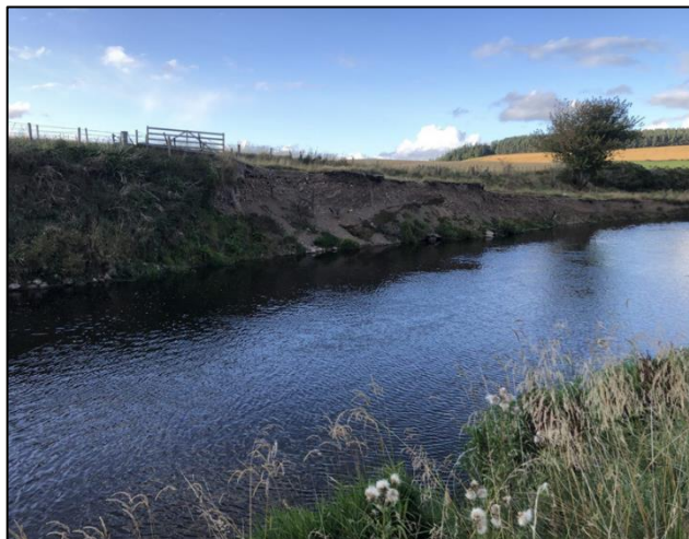
Figure 3.7. Bank erosion on the river left bank at Jock Reid pool, just upstream of the embankment breach area.
