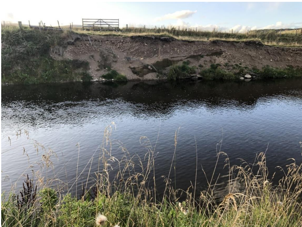
Figure 4.15 Bank erosion between Jock Reid pool and the breached embankment. The track was previously positioned between the gate/fence line and the top of the channel bank, however this route is no longer safe to access due to the erosion and embankment breach. Bank height within this section ranges from 1 to 3 m.
